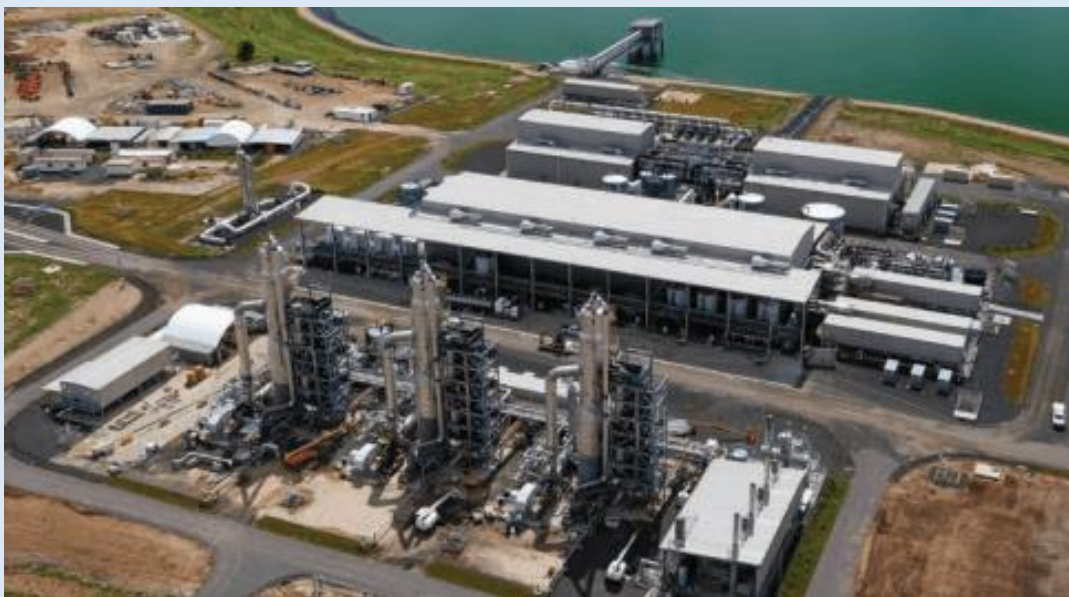
Figure 19 - QGC's Wooleebee Water Treatment Plant
